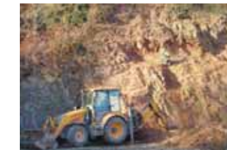
Contractors working on a conservation project in a former-diorite quarry at Parley, near Nuneaton.
