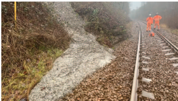
The ‘slow slip’ at Darton began like this, but got worse over a number of hours. (Image: Network Rail)
