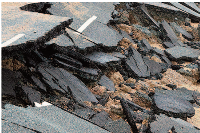
This was the A379 at Torcross, it will have to be completely rebuilt in a different place.
