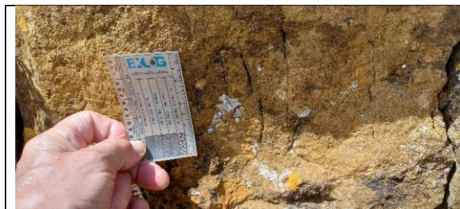
Figure 37: Stress fractures in a Marlstone block
